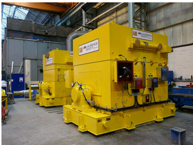
Abb. 1: ATB Laurence Scott Ltd., New inverter drive test facility
